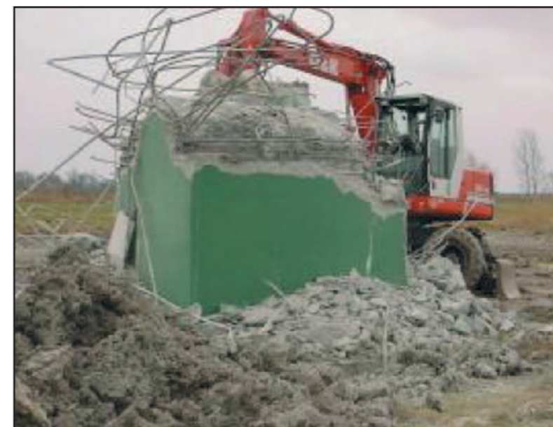
Figure 262: Destruction de la base
